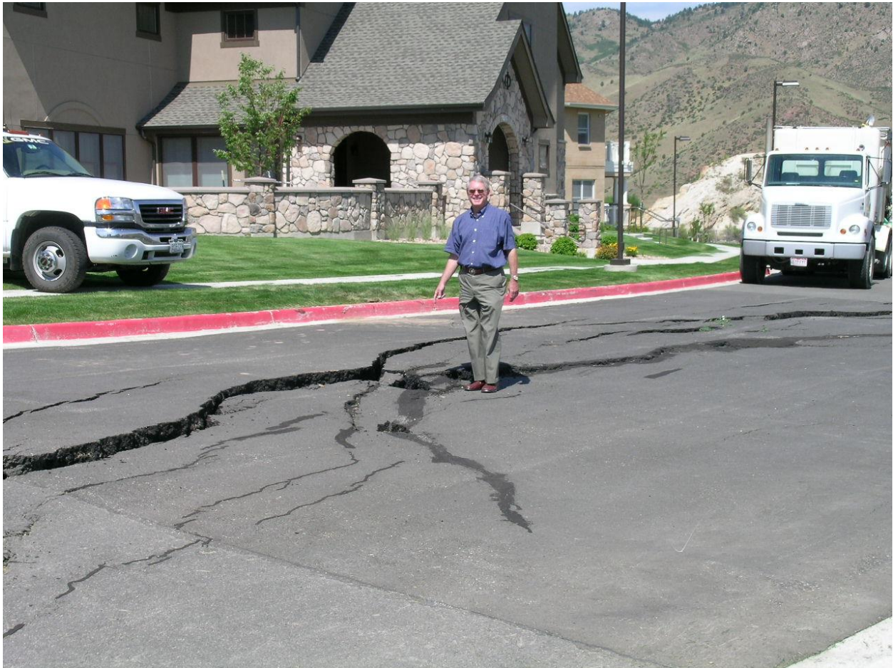
Subsidence is a particular concern for many communities across Colorado. This image from 2005 shows road damage likely initiated by subsidence in Golden near the Colorado School of Mines.
